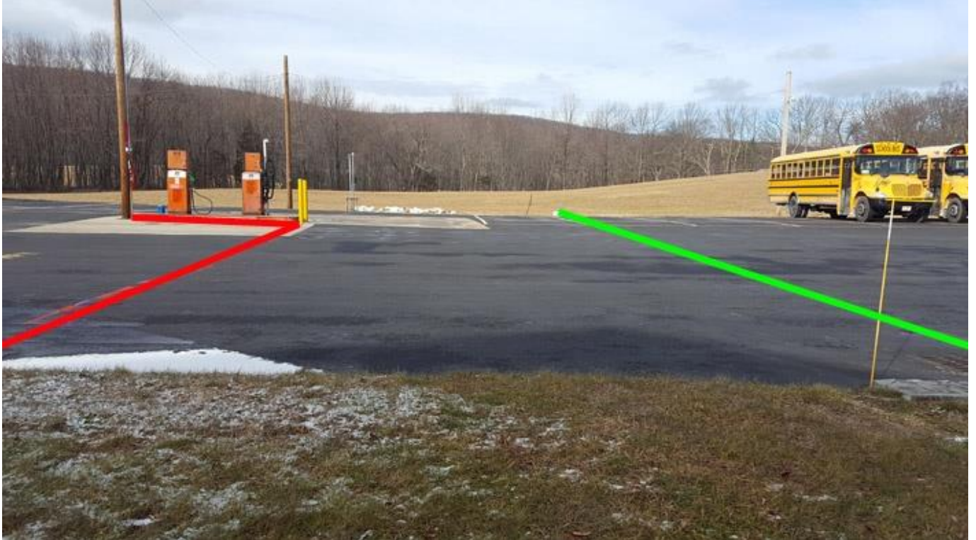
Northwest facing photo of the fueling island area as seen from near the building shows the electric line in red and a storm sewer in green.
