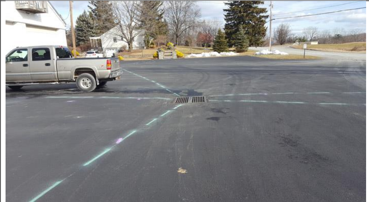
Northeast facing photo of the central sewer grate in front of the bus service building where five separate drains converge.
