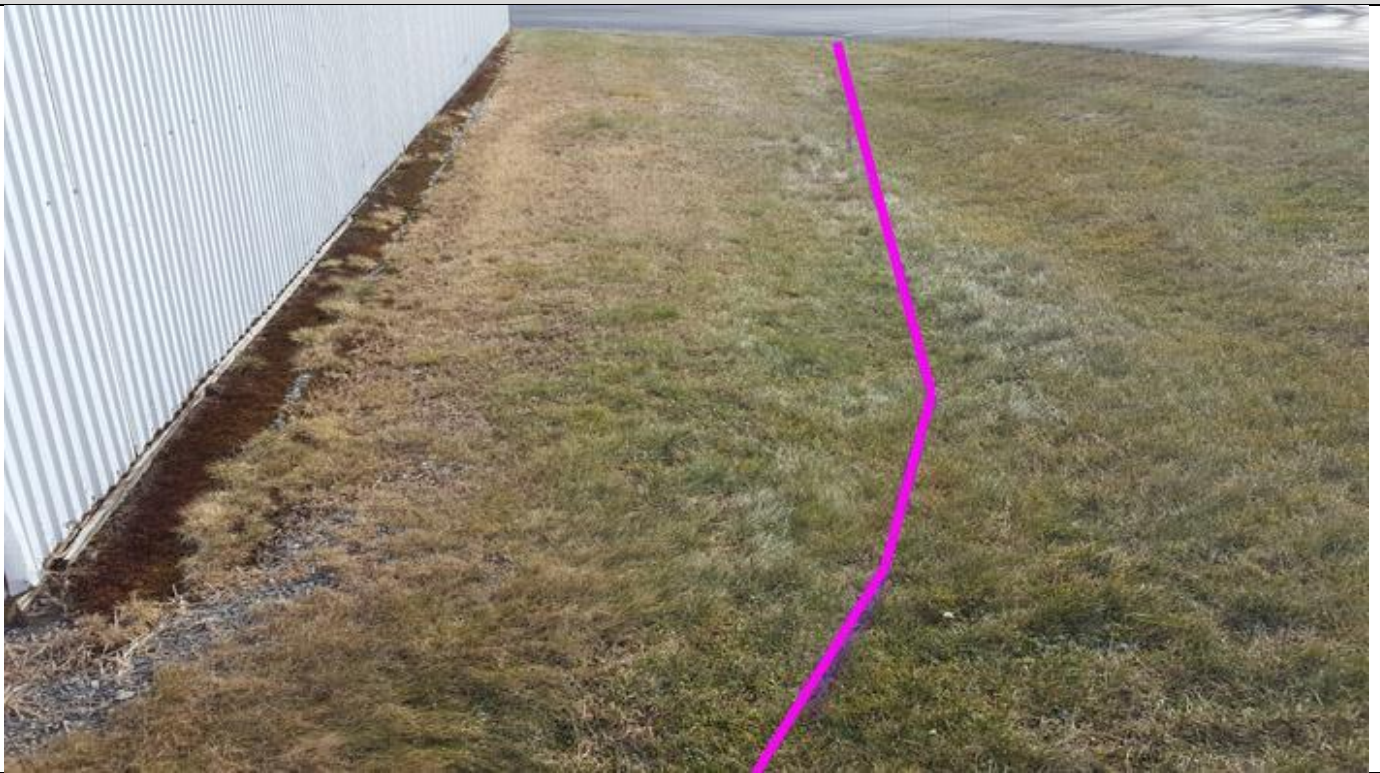
South facing photo shows the path of a zone which appears to be a gravel filled trough that conveys wastewater from the septic system to the storm drain in the distance.
